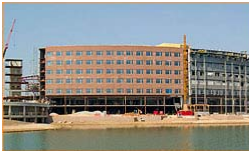
Bringing masonry expertise to the jobsite at the right time “makes the material more relevant and practical,” says Walsh’s training manager.
