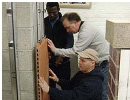
BAC contractors try installing Boston Valley Terra Cotta rain screen wall at the Boston event.
