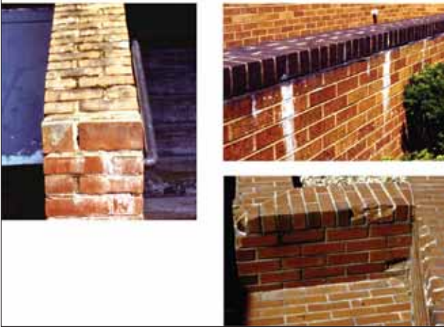
Brick caps are prone to deterioration.
