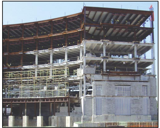
Each of the 14,000 limestone panels required intermediate structural steel framing for support.
