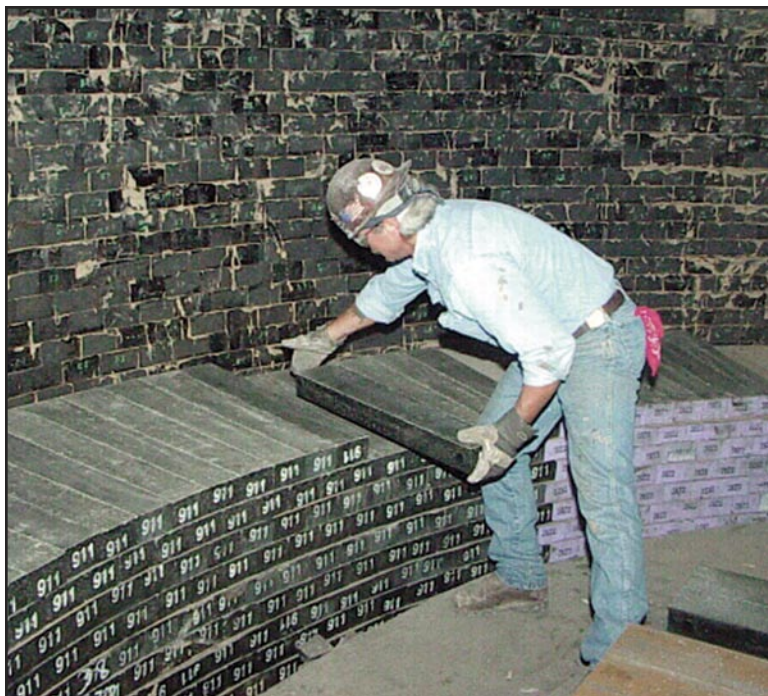
Above: BAC Craftworkers perform a complete brick reline of the #1 BOF vessel.
