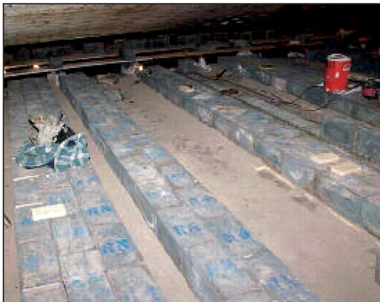
Local #4 Bricklayers replaced four furnace hearths in 2003. The one shown above is located at the 80” Hot Strip Mill.
